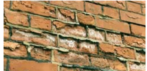
If you want to avoid damage like this then specify Enviro-safe Façade Water repellent.
